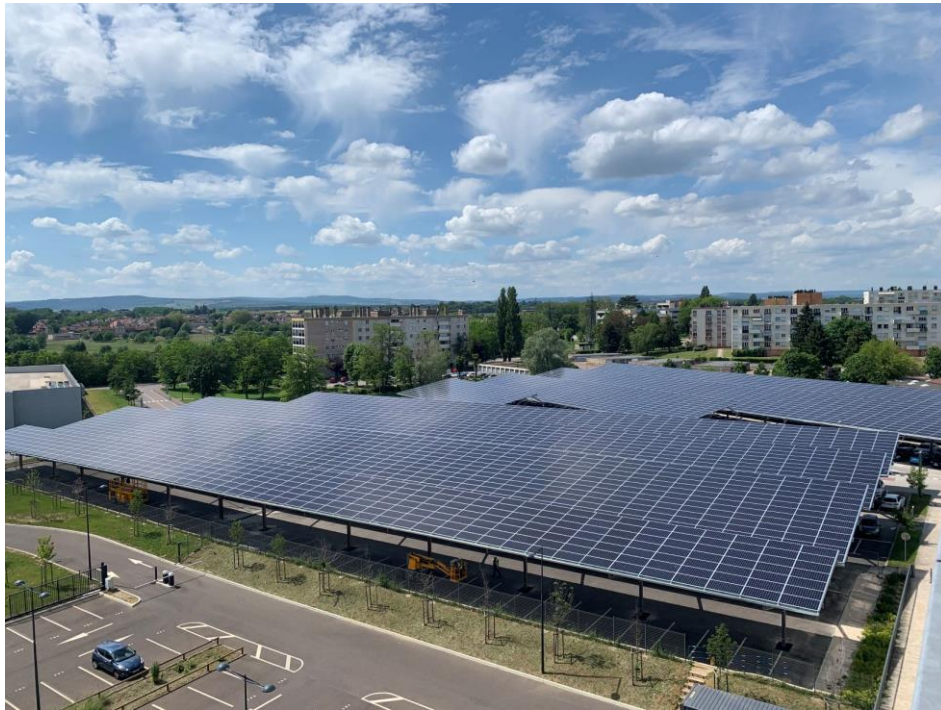
Ombrières photovoltaïques – CH William Morey Chalon-sur-Saône (71)
